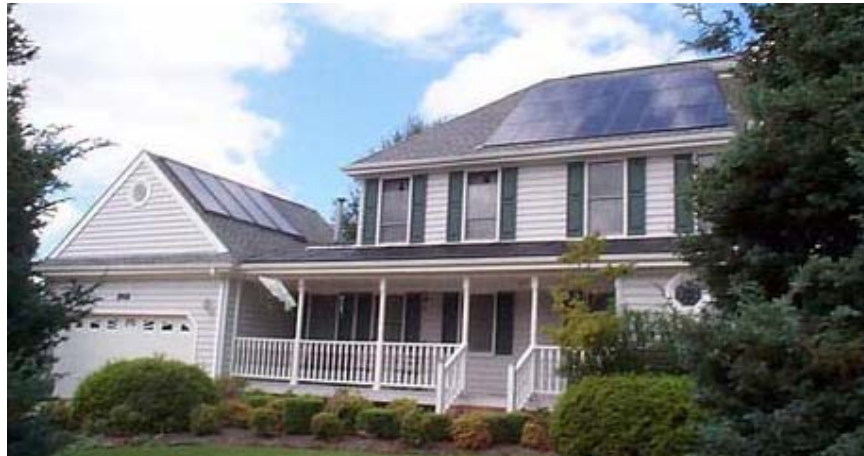
Figure 3. A SOLAR PV ARRAY CONSTRUCTED ON MULTIPLE ROOF FACES, GIVING AN EFFECT SIMILAR TO THAT OF DIFFUSE SHADING.
